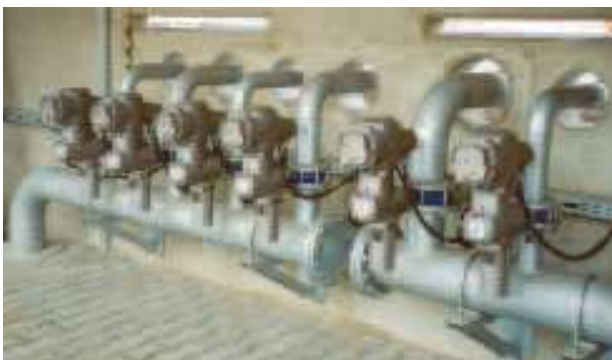
AUMA part-turn actuators with AUMA MATIC integral controls in a tank farm in Poland.
