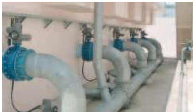
AUMA part-turn actuators mounted to butterfly valves in a Vietnamese water treatment plant.
