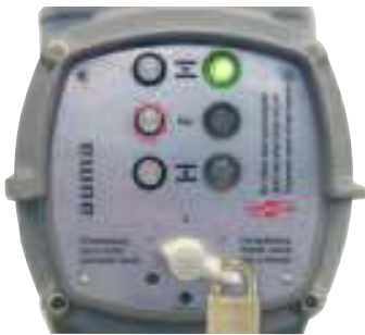
AUMA MATIC local controls with push buttons, selector switches and indication lights
